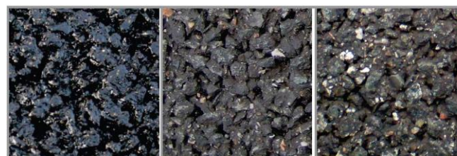
Figure 3. The road surface with a LOA D: a) fresh after paving, b) after 10 months, c) after 19 months, Source: M. Schünemann, 2011
