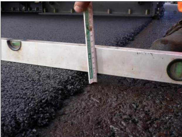
Figure 2. Thin hot mix asphalt overlays on the road seal (DSH-V) uncompacted 18 mm thick, Source: M. Schellenberger, 2010
