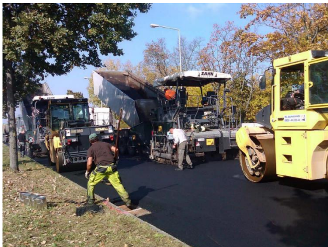
Figure 4. Installation of noise-optimised asphalt wearing course AC 5 D LOA on Rheinbrückenstrasse, Karlsruhe, Germany, Source: M. Schellenberger, 2010
