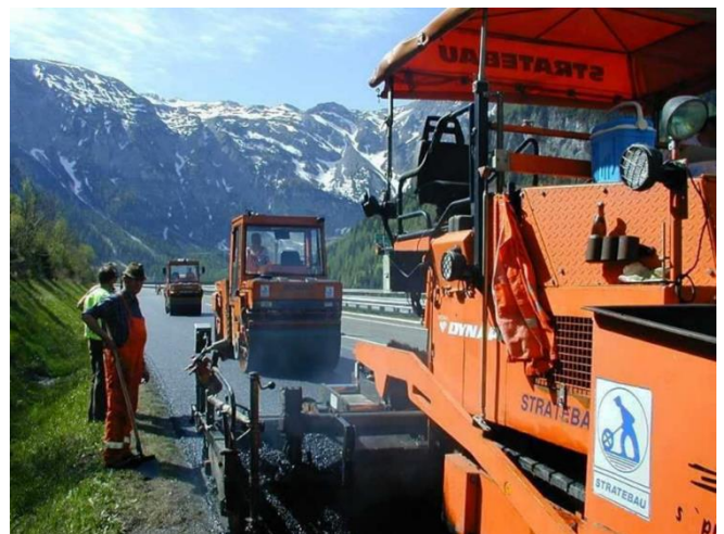
Figure 9. Installation of noise-reducing SMA LA asphalt on the A10 Tauern motorway in Austria in May 2003, Source: K. Graf, M. Schellenberger, 2009
