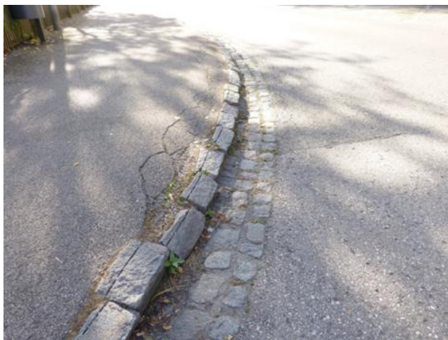
Figure 14. Example of kerb displacement and detachment of thin asphalt layers
