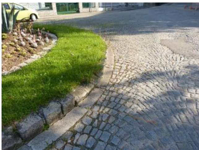
Figure 15. Example of kerb displacement
