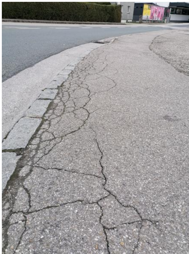
Figure 11. Insufficient joint-filling material at the kerb and cracking in the asphalt footpath Source: Hrapović, 2025
