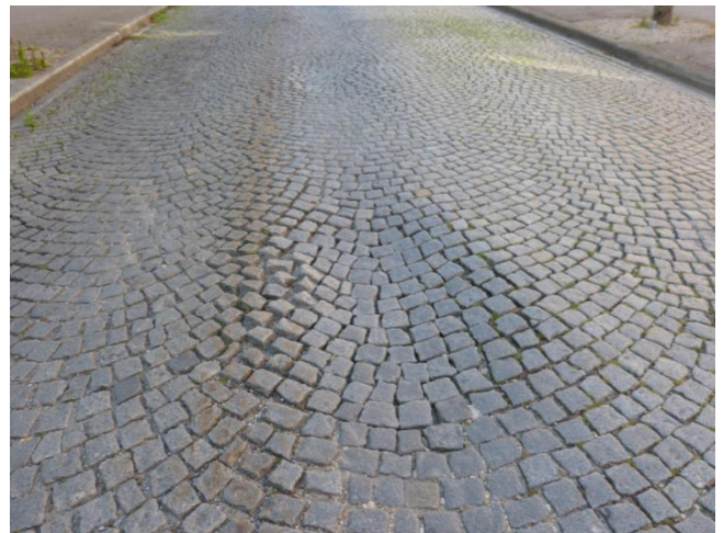
Figure 26. Rutting Source: Hrapović, 2025
