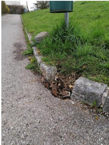
Figure 13. Example of kerb displacement and detachment of thin asphalt layers
