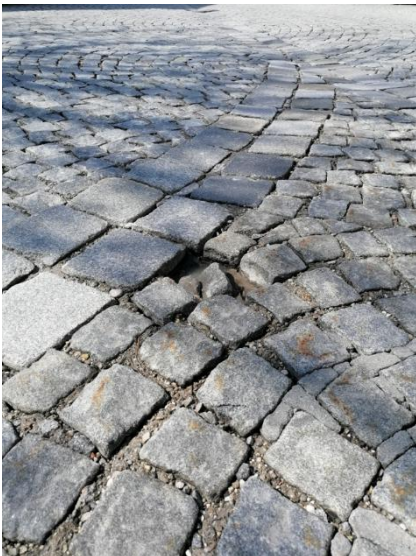
Figure 23. Open joints and tilting of cobblestone elements Source: Hrapović, 2025
