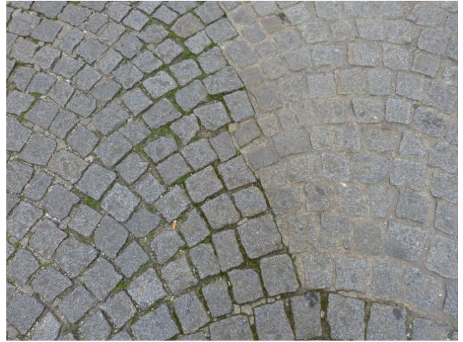
Figure 31. Partially grouted joints filled with mortar Source: Hrapović, 2025
