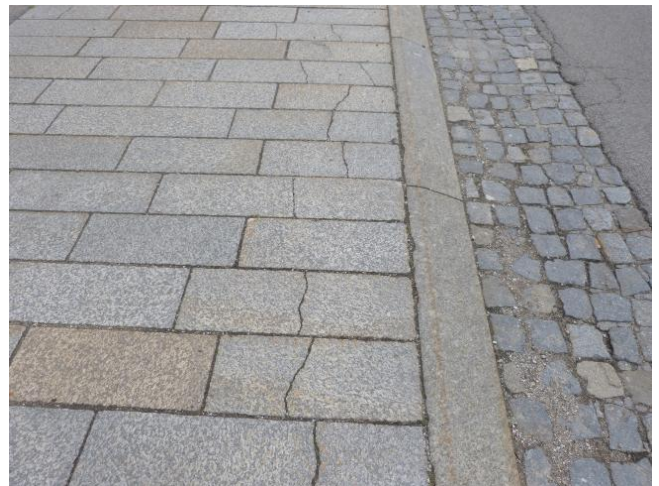
Figure 32. Cracked granite slabs Source: Hrapović, 2025
