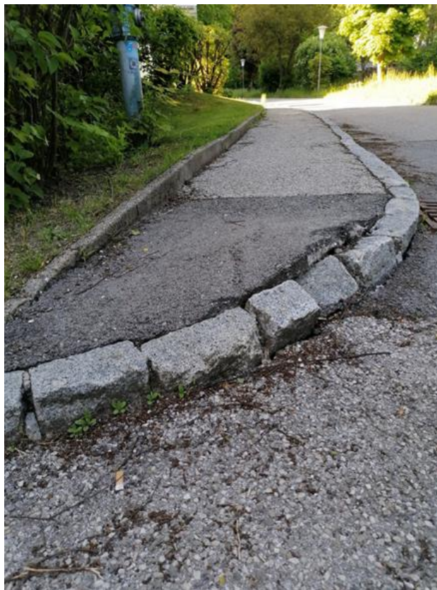
Figure 12. Irregular and poorly executed patch repairs on the footpath
