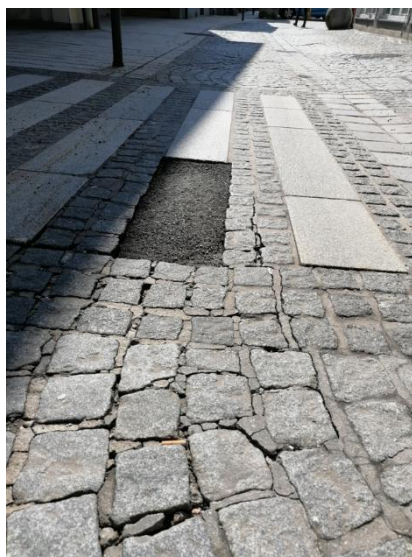
Figure 20. Asphalt-filled patches on a paved surface Source: Hrapović, 2025
