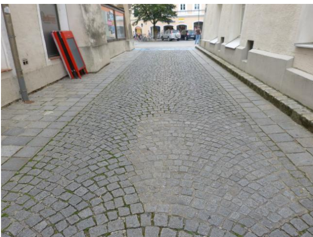
Figure 30. Partially grouted joints filled with mortar Source: Hrapović, 2025
