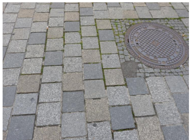
Figure 27. Open joints between slab elements Source: Hrapović, 2025
