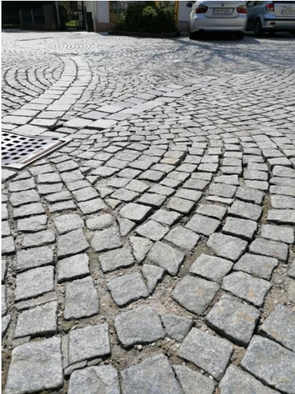
Figure 22. Open joints and tilting of cobblestone elements Source: Hrapović, 2025
