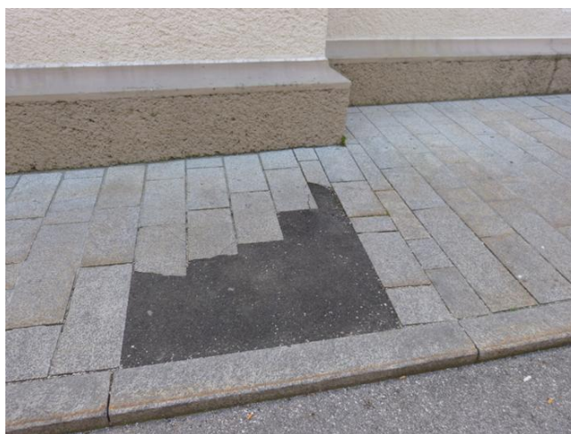
Figure 21. Asphalt-filled patches on a paved surface Source: Hrapović, 2025
