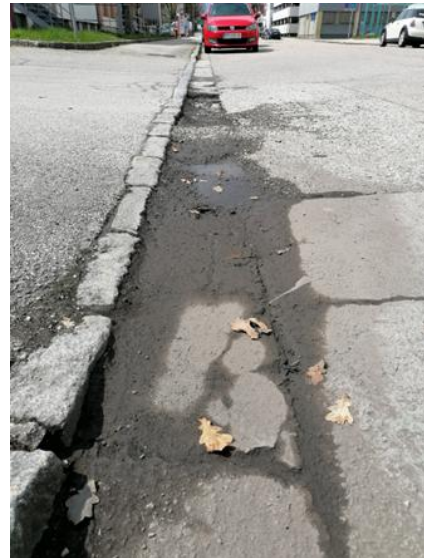
Figure 16. Settlement with cracking in the drainage channel area
