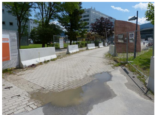
Figure 33. Irregular settlement of cobblestone and asphalt elements Source: Hrapović, 2025
