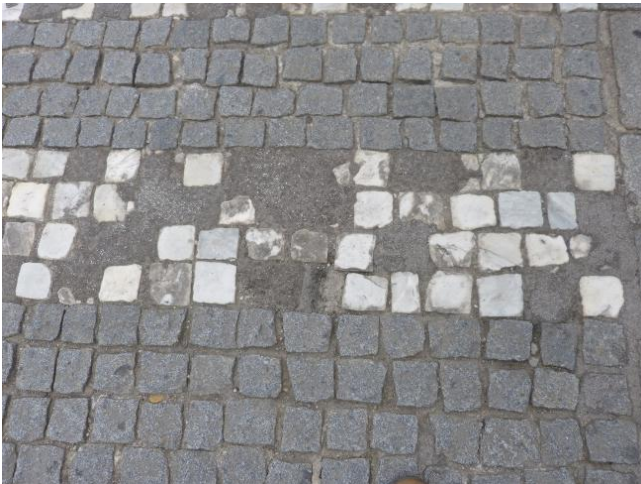
Figure 29. Asphalt-filled patches at a pedestrian crossing made of marble and granite cobblestones Source: Hrapović, 2025
